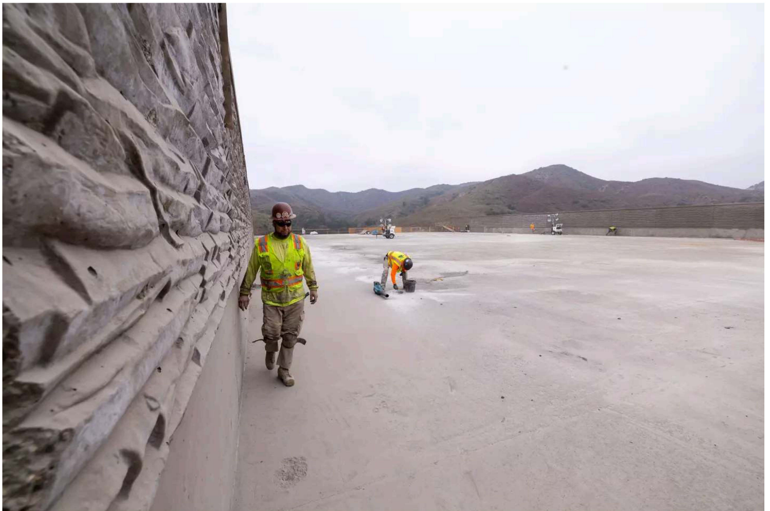
Workers prepare the deck for waterproofing on the Wallis Annenberg Wildlife Crossing in Agoura Hills. (Brian van der Brug / Los Angeles Times)
