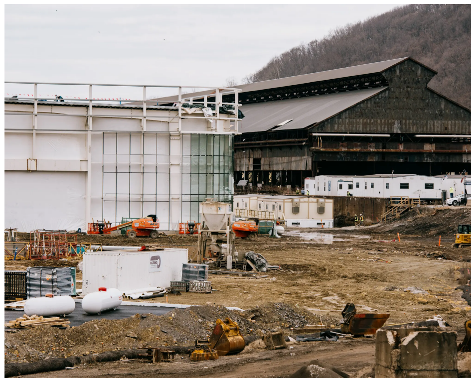
Form Energy's factory is being built on the site of a former steel plant. Kristian Thacker for The New York Times
